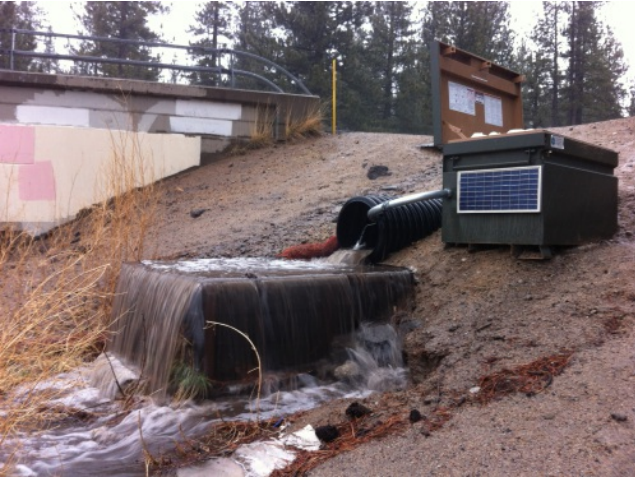
Stormwater monitoring station at the Upper Truckee River site
