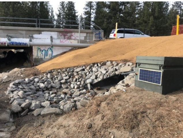
Stormwater monitoring station at Upper Truckee River site after installation of treatment vault.
