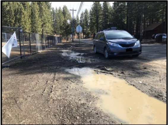
Flooding in parking and pedestrian access area
