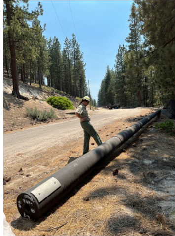
LTBMU Forest Supervisor Erick Walker attends site visit for a system hardening (pole replacement) project at Ponderosa Ranch
