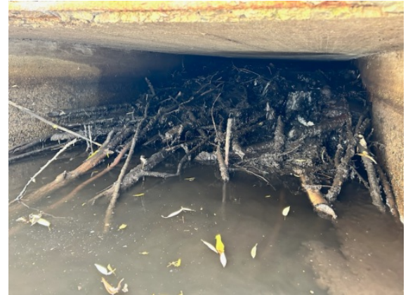
beaver dam within 4ft wide NDOT HWY50 culvert, November 2024
