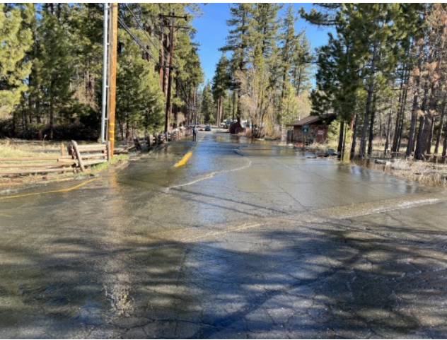
Undersized culvert on Zephyr Cove Resort property creates road flooding, November 2024
