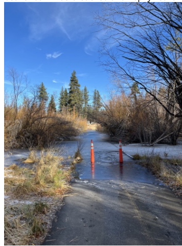
Zephyr Cove Campground Trail flooded due to beaver dam in NDOT HWY50 culvert, November 2024
