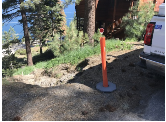
Slope erosion resulting from failing timber retaining wall at Beowawie
