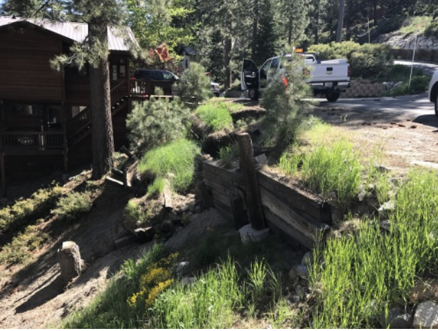
Failing timber retaining wall at Beowawie
