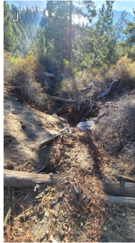
Eroded ditch due to undersized stormwater infrastructure
