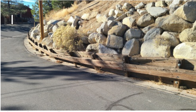
Failing wood retaining wall
