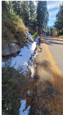
stormwater runoff creating erosion and threatening road integrity
